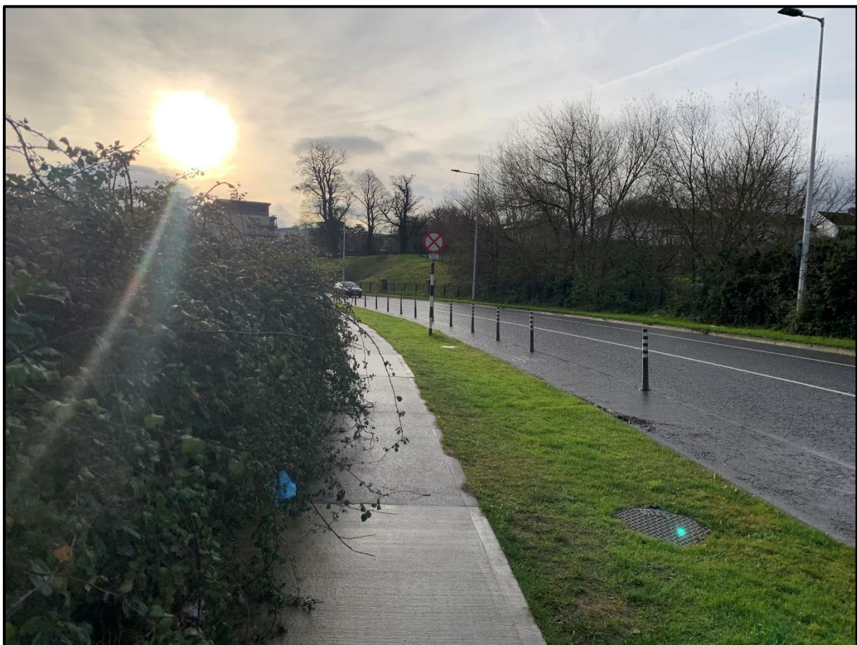
Figure 3.4: Overgrown vegetation along the footpath edges
